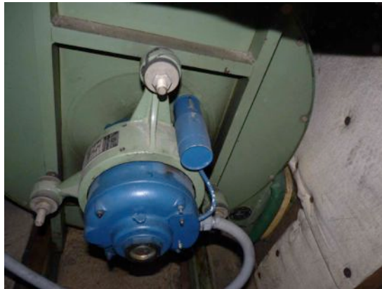
(L) blower fan case and replacement motor
