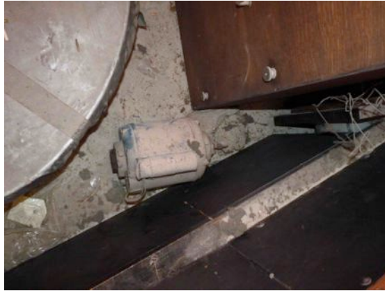
(L) original blower motor plus debris
